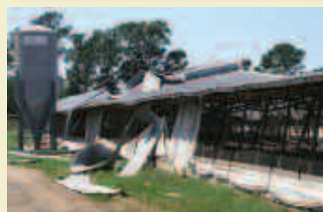
A house in St. Tammany Parish in Louisiana and a poultry house on a farm in Mississippi suffered severe damages from the recent Gulf Coast hurricane. Farm Bureau insurance companies work together when catastrophes like the hurricane strike.
